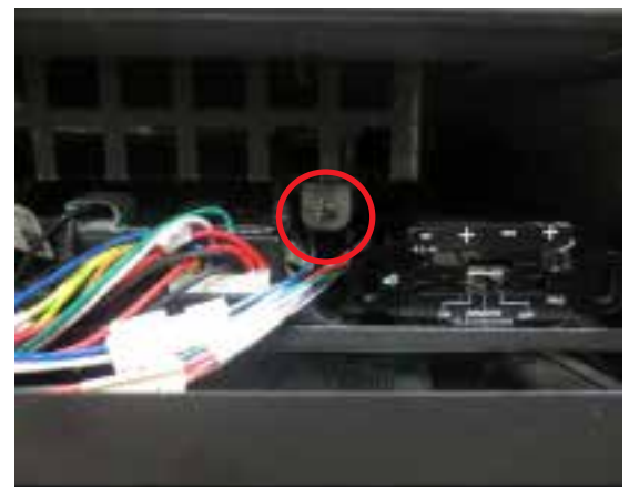
The Surefire switch is located at the bottom right above the DFC board.
