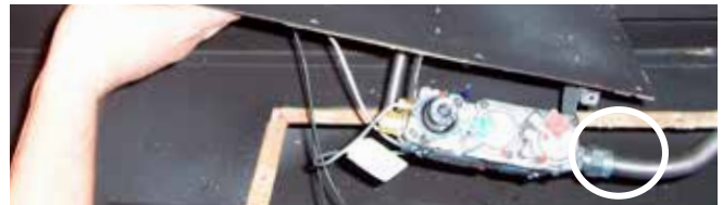
Gas Inlet Line
