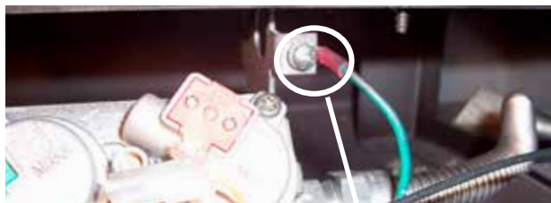
Green ground wire
